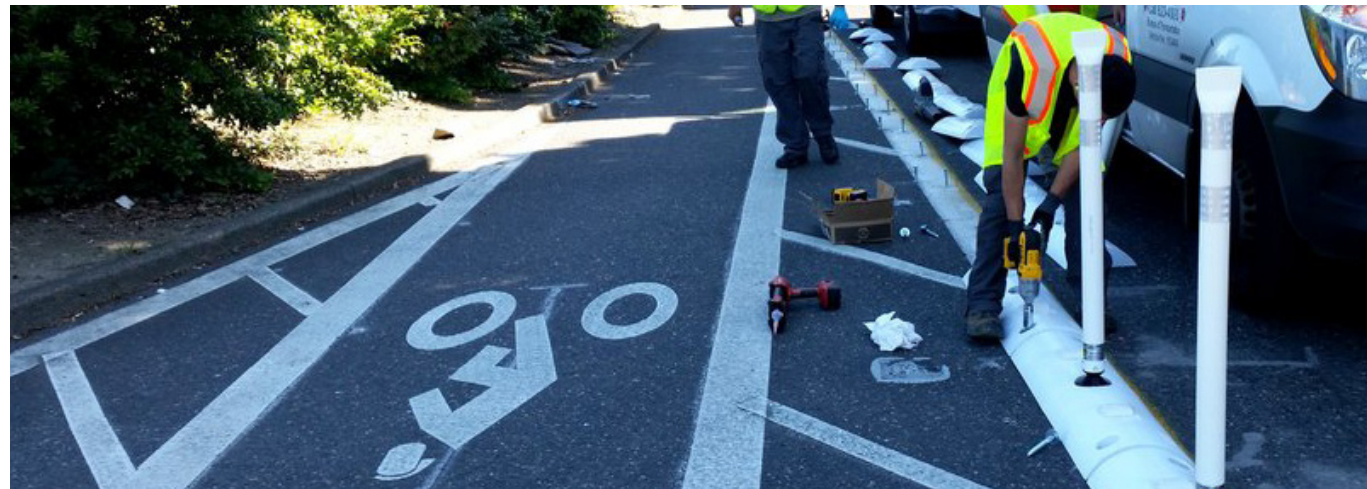
Top left: Flexible delineators proved ineffective at SW 13th Avenue and Clay Street (Jonathan Maus, Bike Portland); Top right: Raised lane separators provided a more robust barrier between people driving and people cycling (City of Portland Bureau of Transportation); Bottom: Raised lane separators are bolted into the asphalt (City of Portland Bureau of Transportation).
